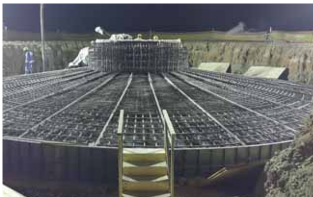
LOERIESFONTEIN WINDFARM, NORTHERN CAPE
